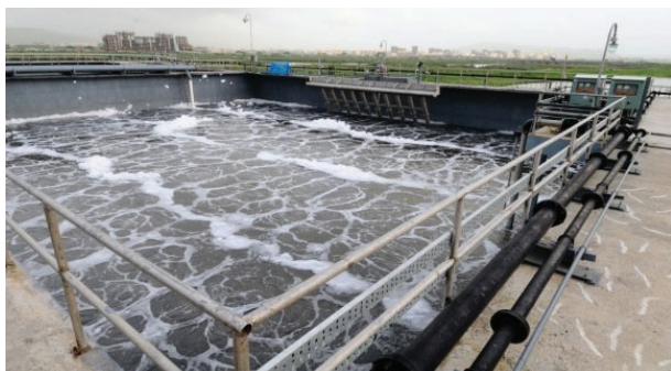
Figure 22.4 A view of sewage treatment plant
