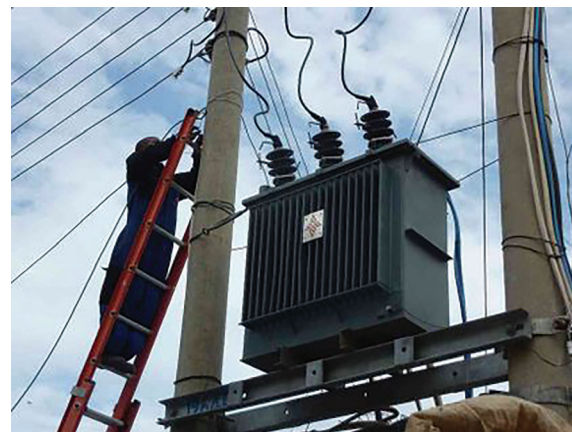
Figure 4.32(b) Roadside transformer
