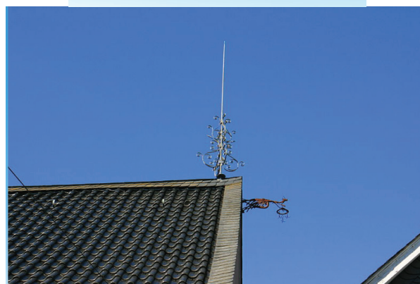
Figure 1.62 (a) Schematic diagram of a lightning arrester. (b) A house with a lightning arrester
